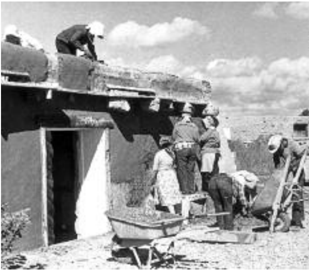
Plastering a home in Llano Quemado, south of Taos, New Mexico, 1966. Photo by Mildred T. Crews, Courtesy Palace of the Governors (MNM/DCA), #066644.
